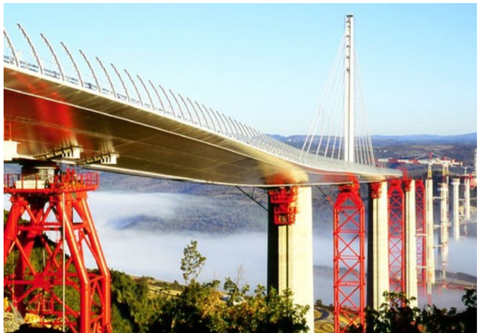
Construction Photos of Millau Bridge in France, World’s Highest Bridge Courtesy of darkroastedblend.com
